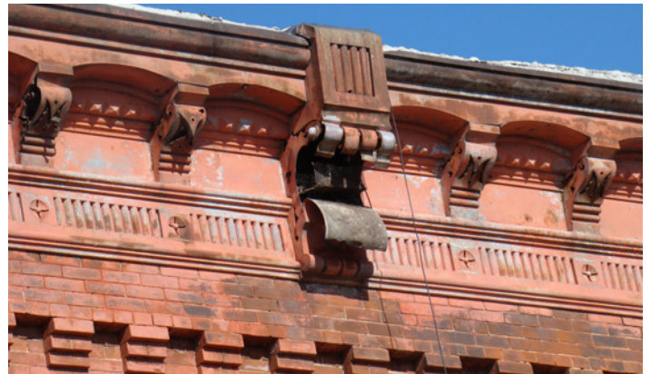
Metal cornices should be painted, and missing or damaged pieces should be repaired.
